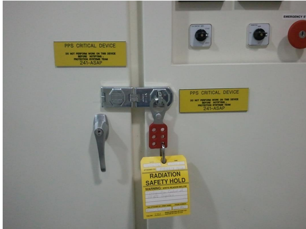
Four PPS Controlled Power Supplies 1 in HEBT, 2 in RSB, and 1 in RTBT
