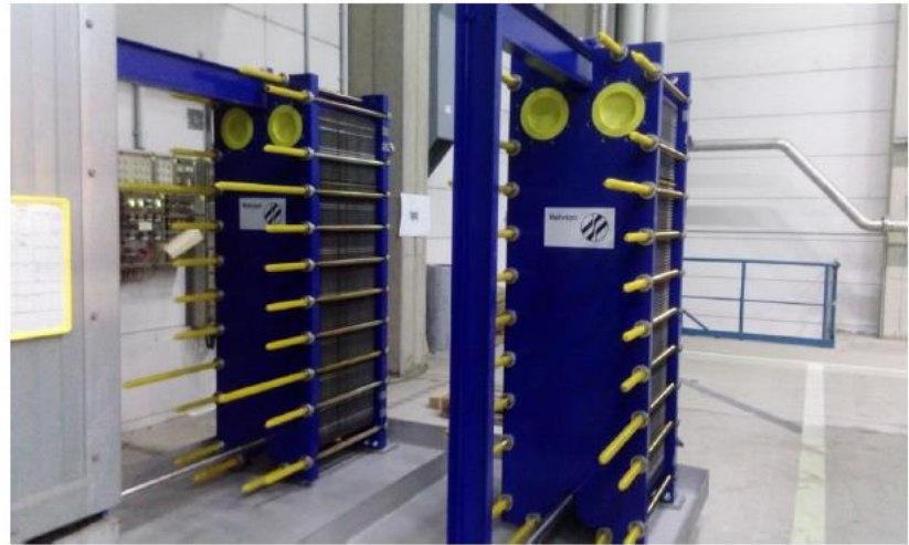
Oil-water heat exchanger
